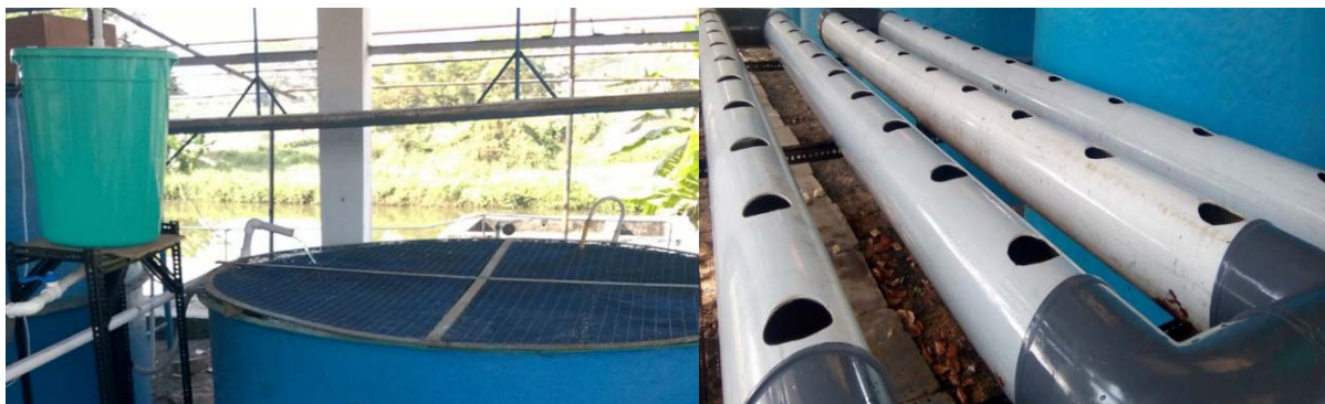
Fig 2: The Aquaponics system setup. A. Fish tank and trickling filter B. NFT grow pipes
